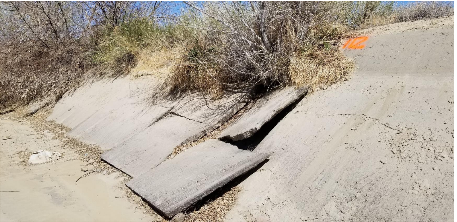
Hogback Canal Lining Rehabilitation Phase II Typical Condition
